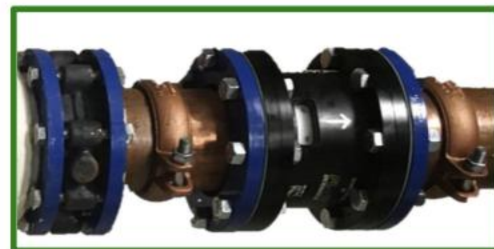
6" Smart Water Valve Installed at Houston Hospital
